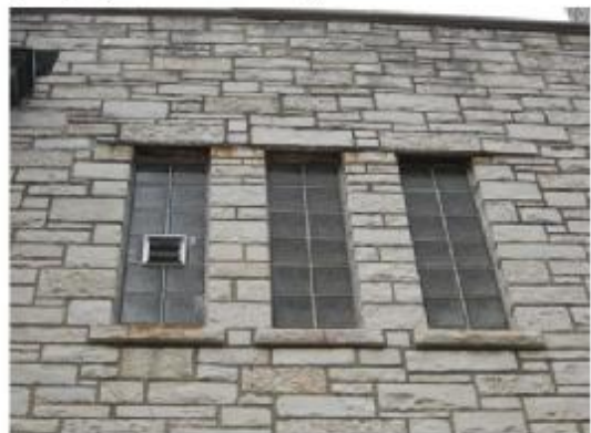
Lintel rusting expansion due to water from parapet: note bowing out, cracking of masonry
