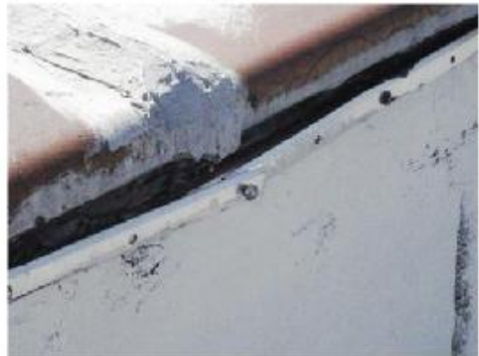
Wood termination bar failure admits water to parapet (see results below)
