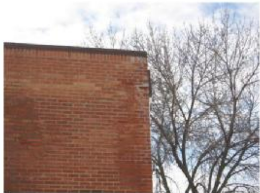
Note soaking and water of brick at corner due to poor flashing and/or scupper design
