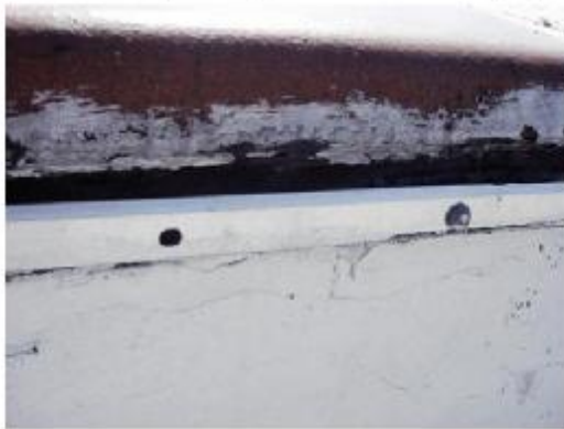
Wood termination bar for roofing at parapet. An inferior installation
