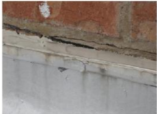
Note extended crack in brick joint resulting in ceiling damage in three rooms below
