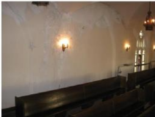
Note extent of sanctuary plaster damage due to poor flashing at parapet—since repaired.
