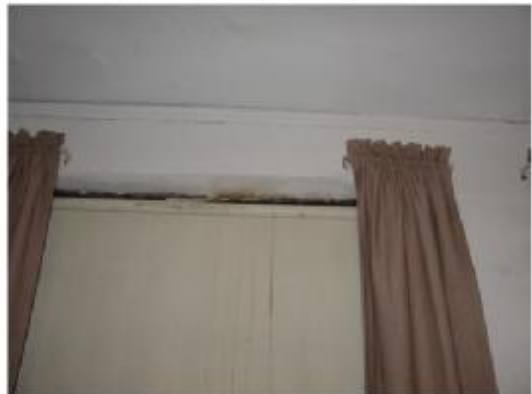
Note rusting lintel at top of window due to failure of flashing and open brick joints at roof above
