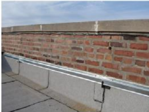
Flat roof flashed to brick parapet— good example with metal cap flashing, membrane under coping
