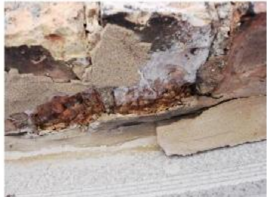
Brick parapet completely disintegrated from water penetration and freezing
