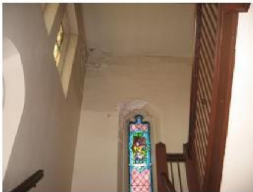
Note plaster damage at ceiling and stained glass window due to flashing failure above
