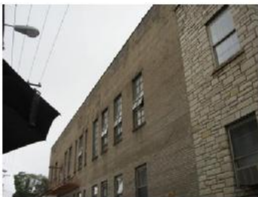
Note dark patches on brick indicating soaking from water penetration in the parapet
