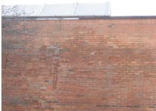
Note open brick joints and ice forming from water in the parapet and wall below
