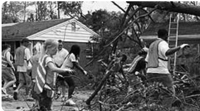
PDA volunteers in North Carolina help survivors clean up debris and do temporary repairs following storms and tornados.
